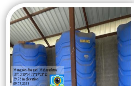
Overhead water tanks
