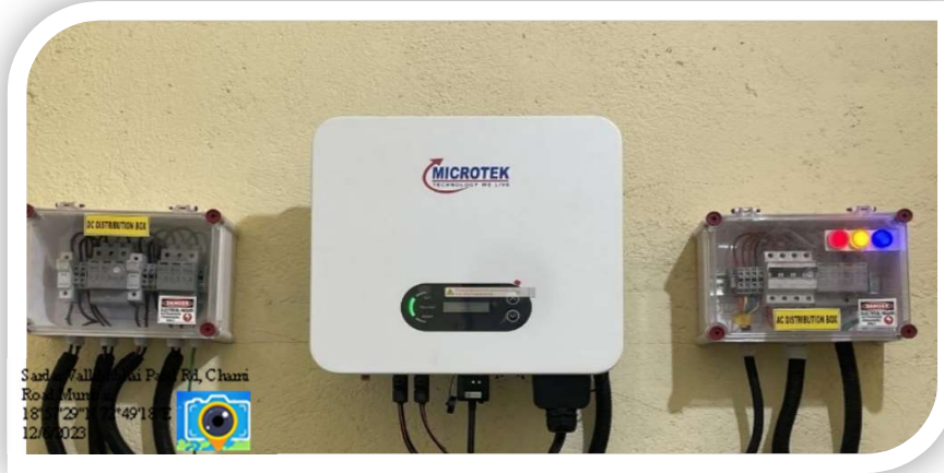
Electric Maintenance equipment's
