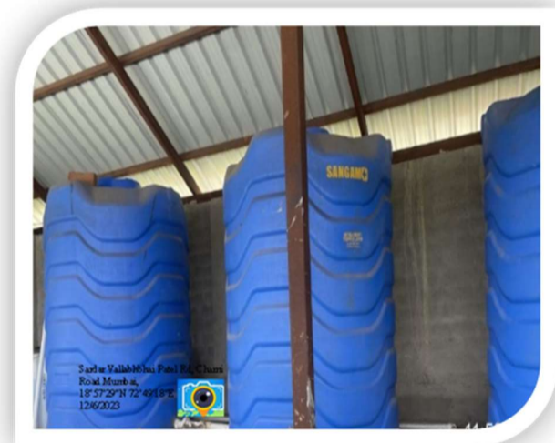
Overhead water tanks
